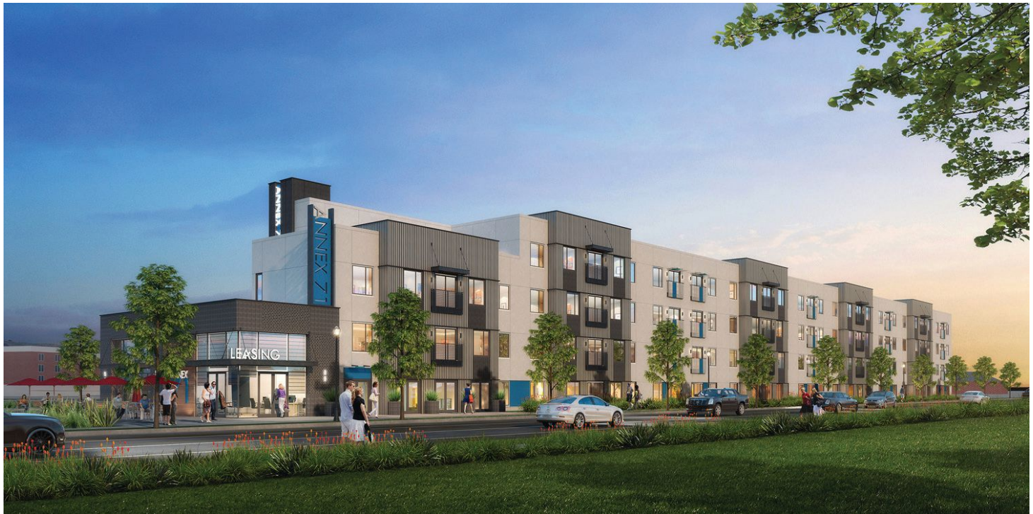
Construction has begun on KTGY Architecture + Planning's project, Annex 71. The residential project will create 140 new residences at the University of Wisconsin-Oshkosh.
